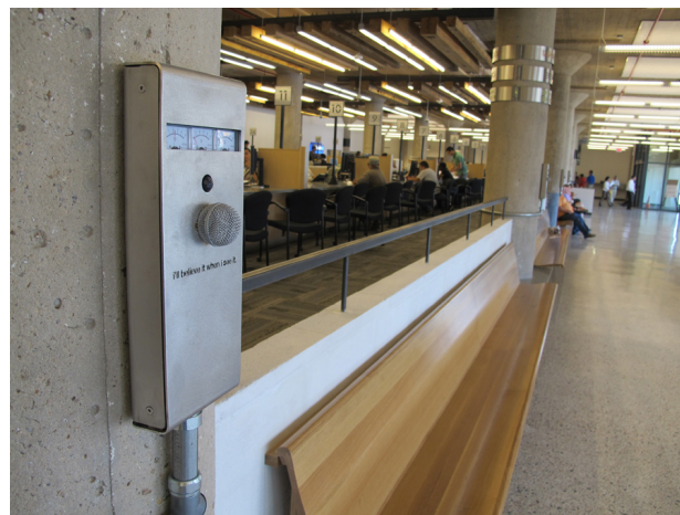
Figure 2. Central Permitting Center waiting area, stainless steel sensor enclosure on existing concrete column
